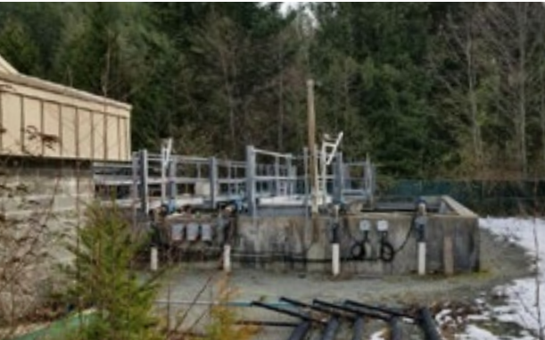
A self-contained treatment plant was installed by the developer and handed over to the SLRD.
