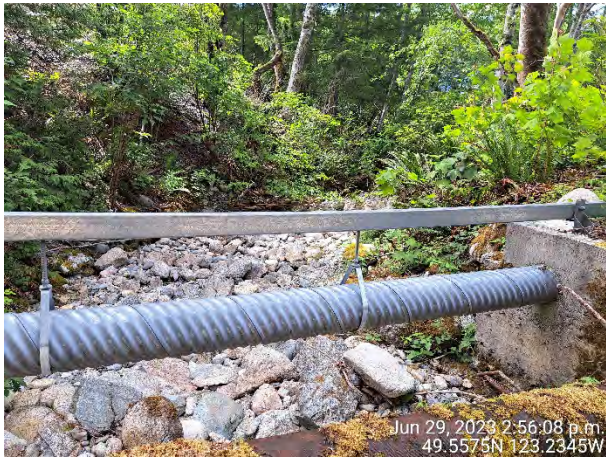
Photo 15: Looking west (downstream) at water pipes crossing Unnamed Stream 1 on the subject site that convey drinking water to the neighbouring provincial park.
