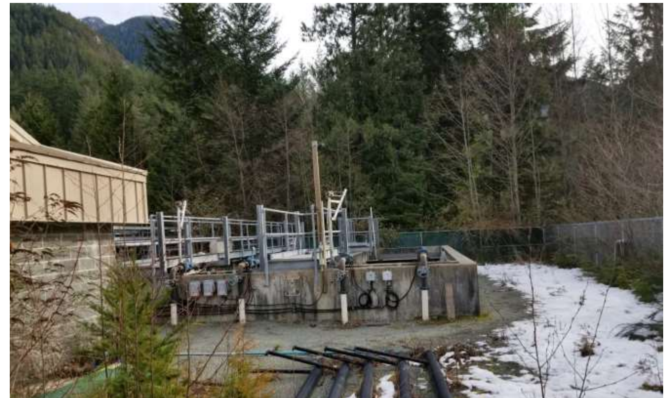
A self-contained waste water treatment plant was installed by the developer and handed over to the SLRD.
