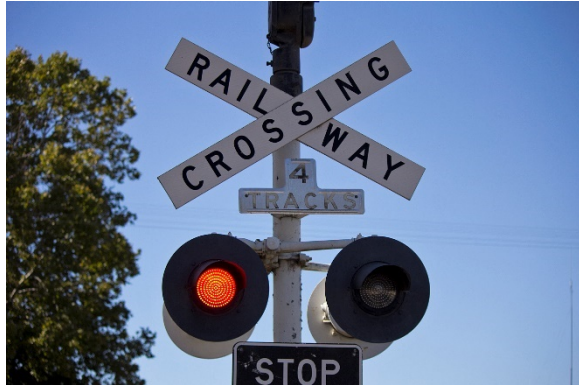
Photo 2: Railway crossing warning systems and barriers
