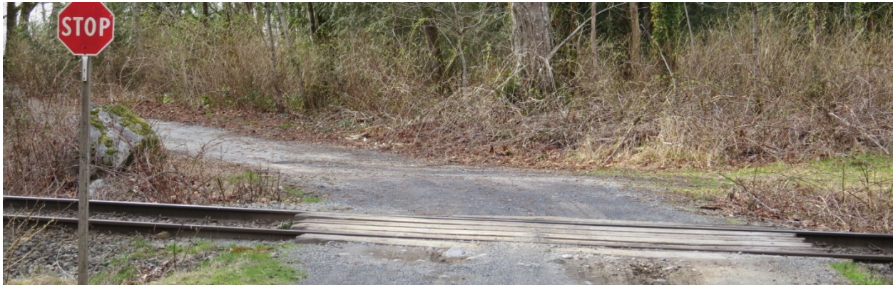
Photo 1: Existing non-conforming CN Rail crossing
