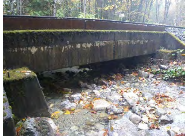
Photo 6: Daisy Creek, looking downstream at railway crossing. Note reduced conveyance due to deposition of sediment.
