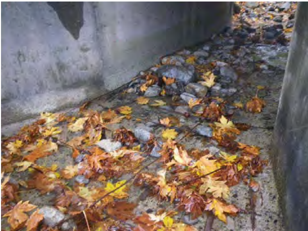
Photo 7: Daisy Creek culvert at ocean. Note poor condition of culvert bottom, with exposed rebar.
