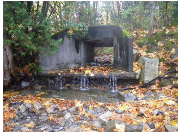
Photo 8: Daisy Creek culvert at ocean, looking upstream. Note drop at culvert outlet.
