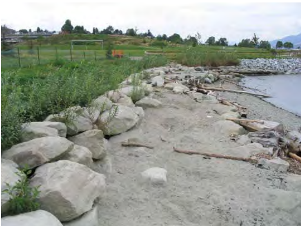
Photo 11: Example of coastal shoreline protection using large rock and plantings.
