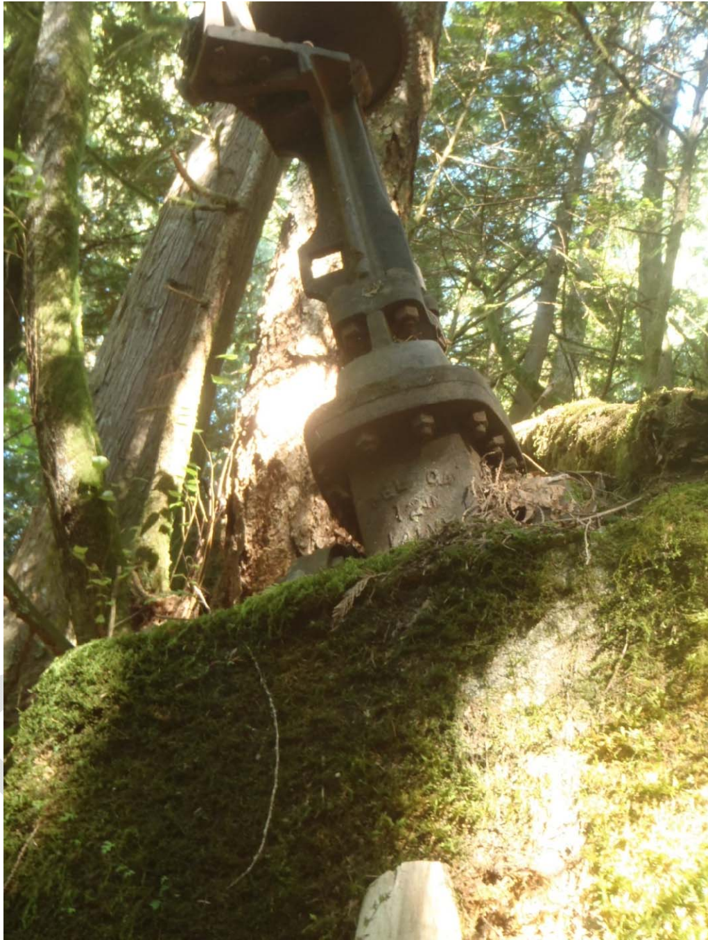
Photo 6. Water control valve in DL 3717.
