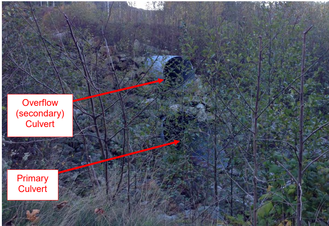
Photo 2: Daisy Creek Debris Basin Culvert Outlet
